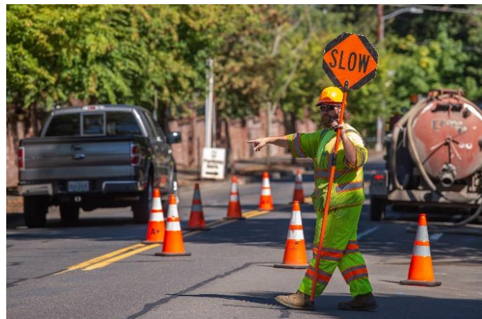
Construction got underway at the Garden Corner Curves in late August and will be completed in 2021.
